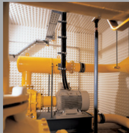
SONEX Pyramid panels used in a manufacturing facility
