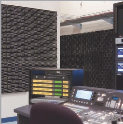
SONEX® Classic Panels in charcoal color tec used in the control room of a broadcast facility
