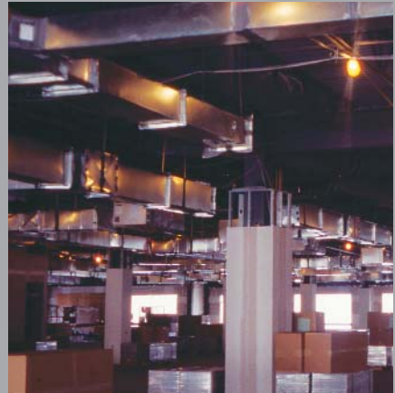
willduct used in ductwork of a manufacturing facility
