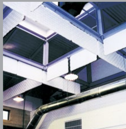
SONEX® One baffles in music room
