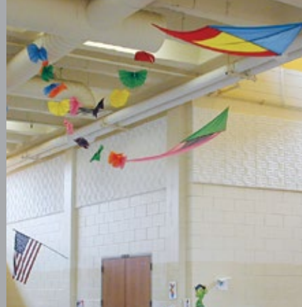
Elementary school's multipurpose room has SONEX® One Panels installed to improve learning environment
