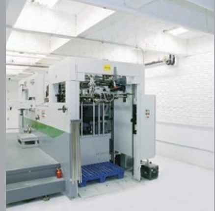
HPC-coated SONEX One Panels help reduce excessive reverberation at printing company
